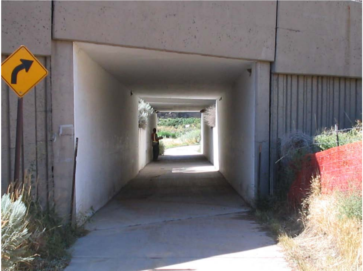
Concrete Box Culvert - This concrete box culvert is one of 5,918 culverts that CDOT inspects regularly. (Photo courtesy of CDOT Staff Bridge.)
