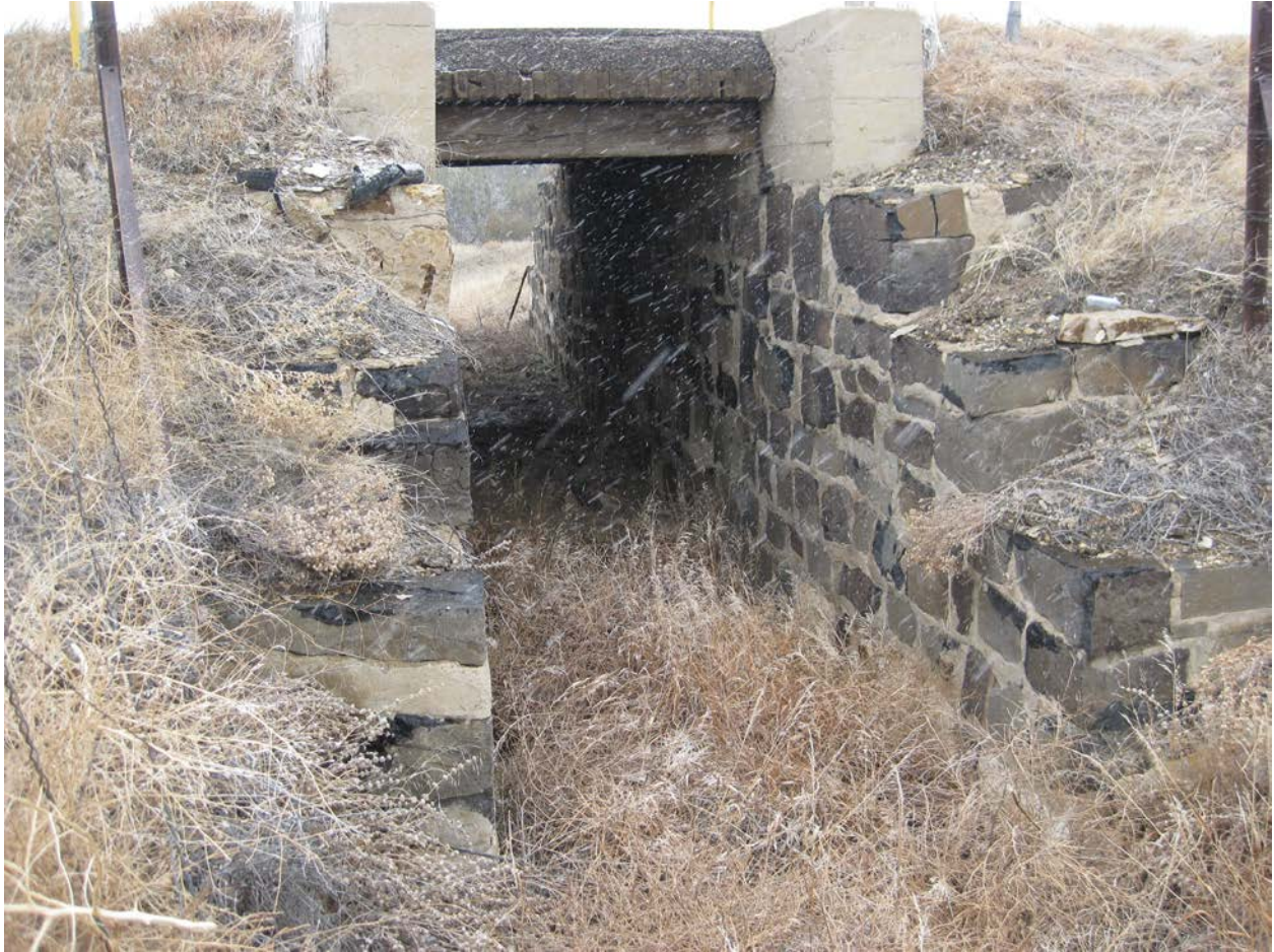
Timber Bridge - This old short-span timber bridge is an example of a minor structure. (Photo courtesy of CDOT Staff Bridge.)
