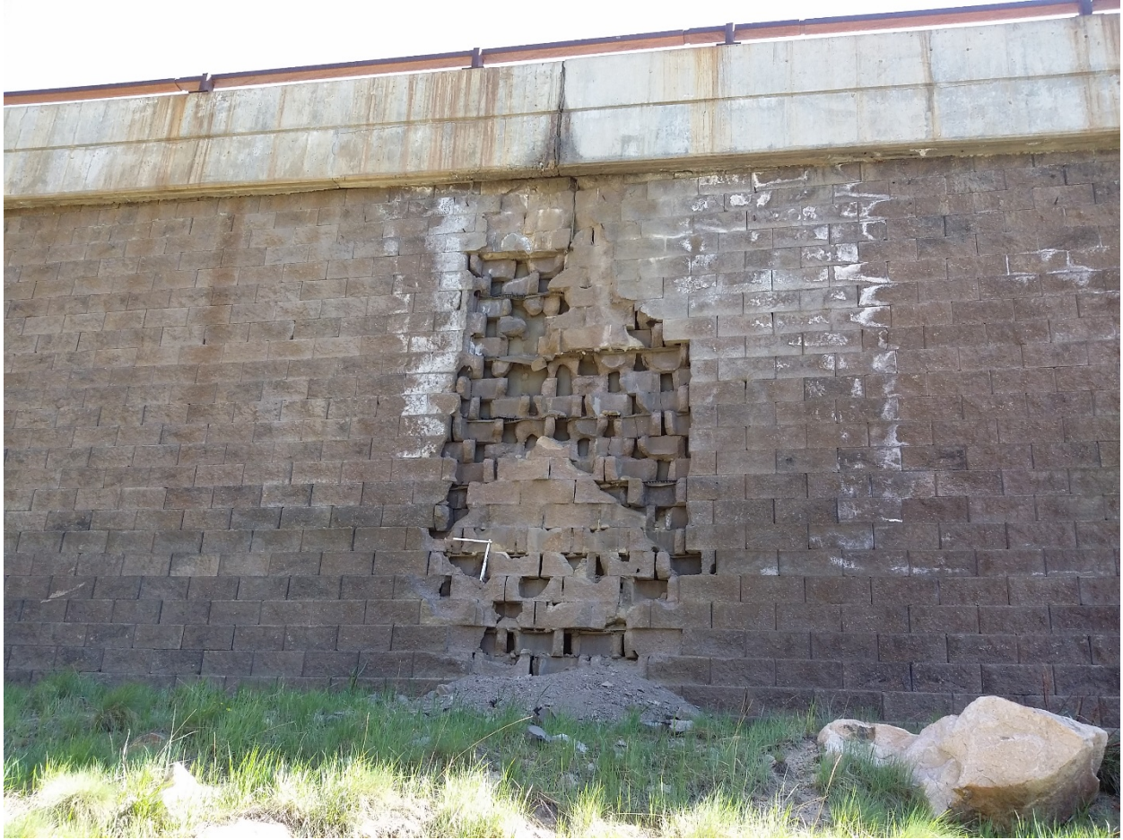
Damaged Wall - Clogged inlets resulted in substantial damage to this wall on Berthoud Pass, which highlights the importance of maintenance activities. (Photo courtesy of CDOT Staff Bridge.)
